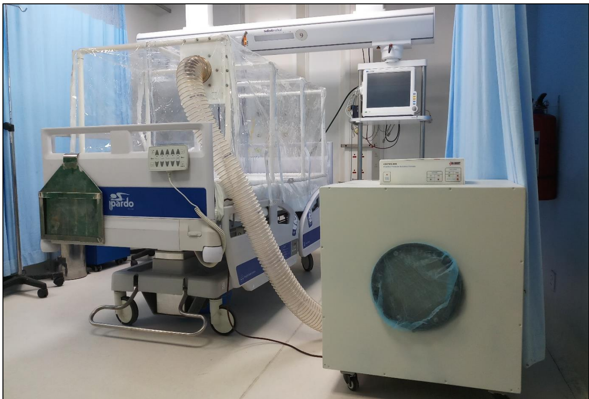
Figure 20. Positive Pressure Isolation Canopy, designed and developed by the author's group, installed at SHNIBPS, Dhaka
