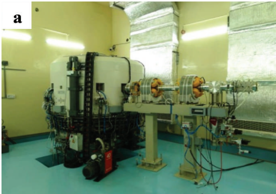
Figure 1: a) Current view of the installed cyclotron at the basement section of oncology building, BSMMU.
