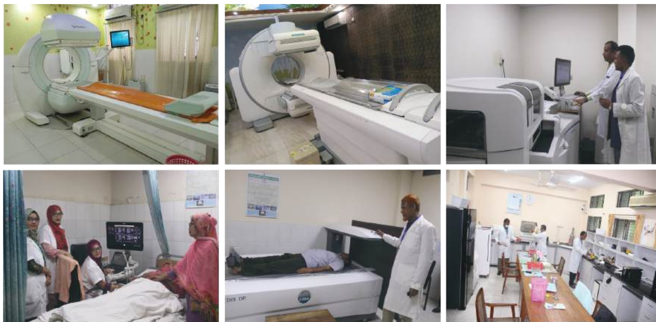
Figure 1: Modern and upgraded nuclear medicine equipment installed at INMAS Rangpur
