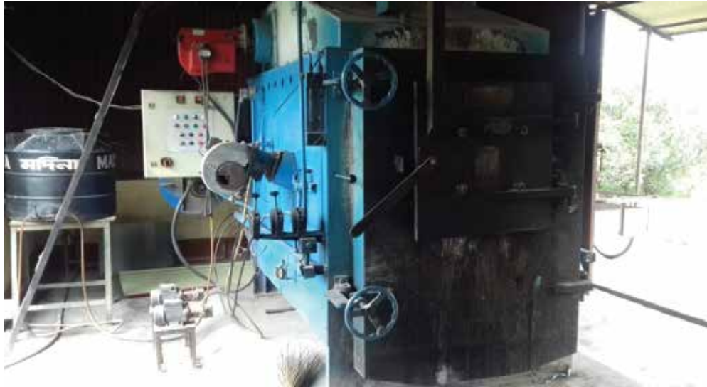
Fig. 1. Incinerator of PRISM Bangladesh at Matuail landfill site
