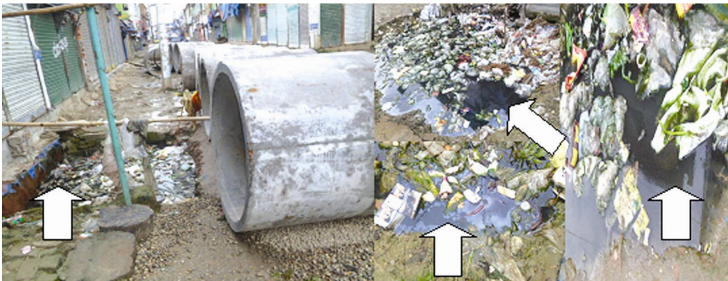
Fig. 2. Under constructing manholes in study site. Arrow signs are showing the mosquito immature density in mosquito breeding sites.
