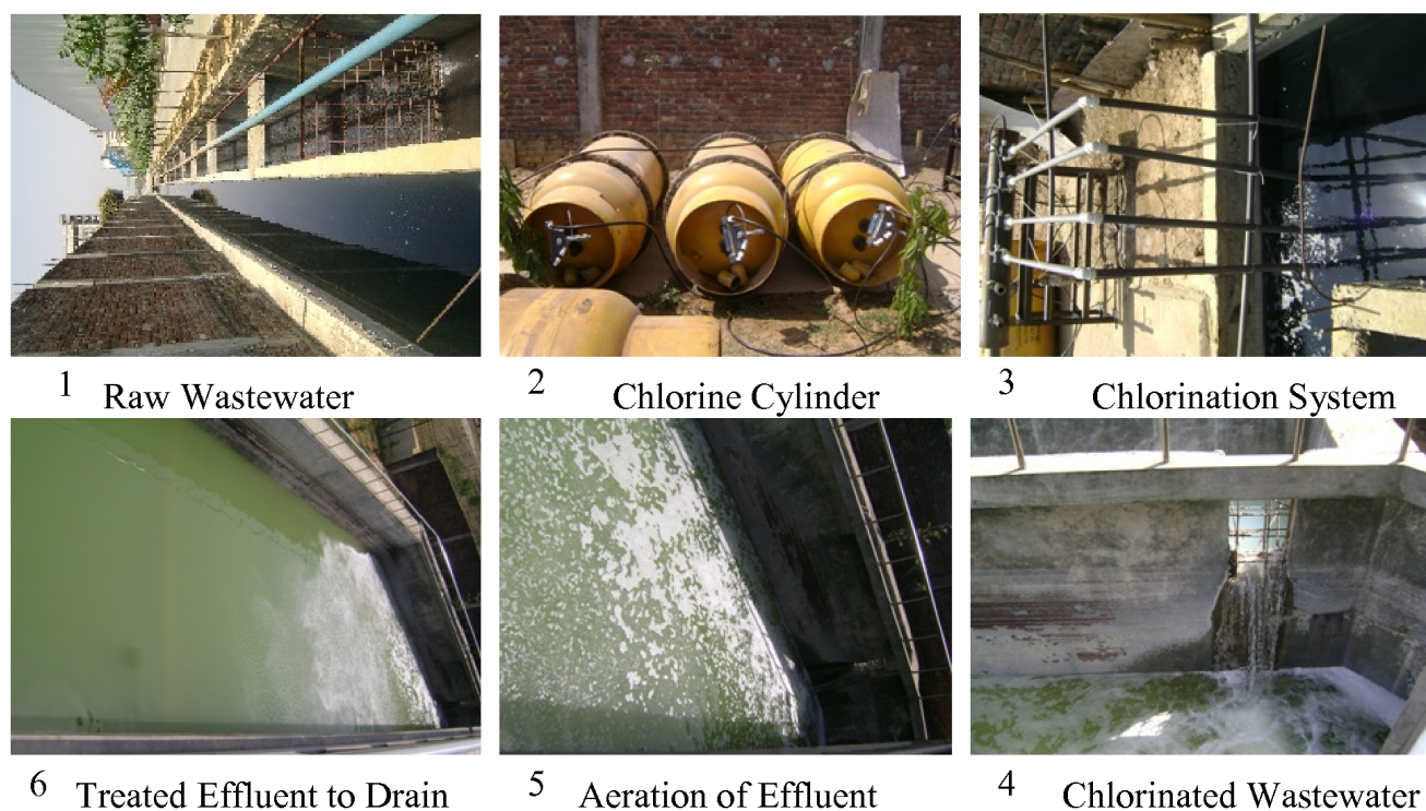
Figure 3: Photograph of a Chlorine based system in a textile processing plant
