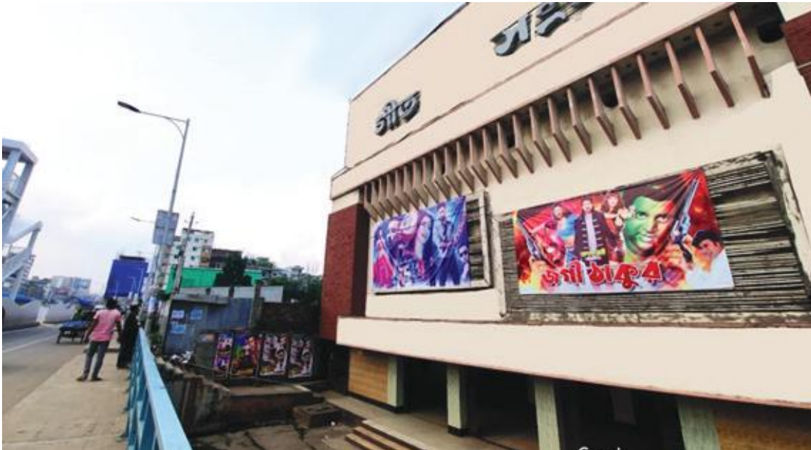
Figure 18: This Picture is Intended to Show How Much the Road was Raised. The Current Road Surface is the One Where the Person in Pink T-shirt is Standing Upon. The Road Surface Used to be at the Same Level as the Entry Way (to the Lower Right Hand Side) of the Geet Sangeet Cinema Hall. A Stairway (Center) now Connects the Hall to the Current Road. (Picture by Akash Ariyan is Collected from Google Maps)
