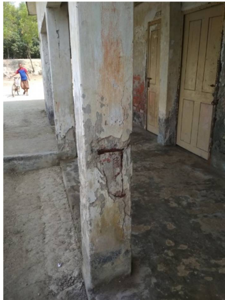
Fig. 4. The extent of structural damage of CS 2 Boro Kupot Primary (81) can be seen to be extreme. The column, which had the load bearing responsibility, has become fragile with the concrete spalling. Moreover, the rods are exposed to air and is rusting away, substantially decreasing their strength.
