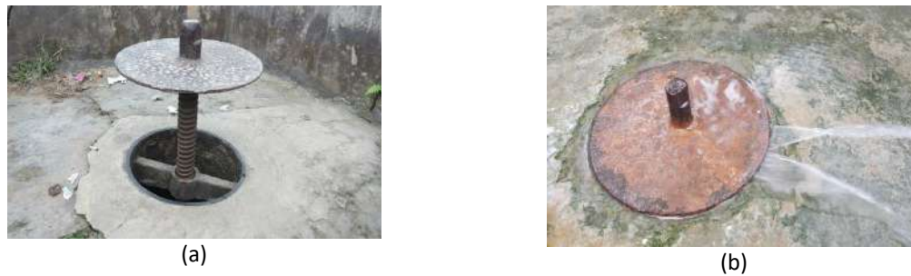
Figure 4. (a) Rust in outlet patches, and (b) water losses through outlet
