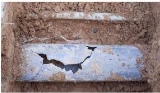
Figure 5. Cracks in the pipe below the ground
