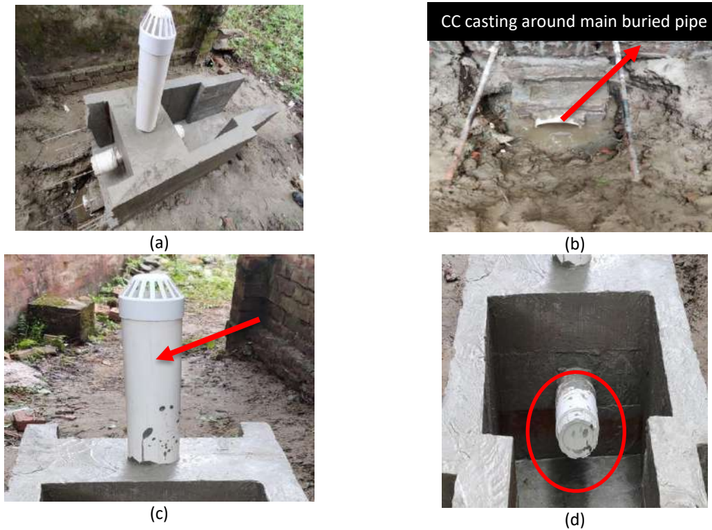
Figure 9. (a) Modified RCC riser outlet, (b) buried pipe within CC structure, (c) newly positioned air vent with strainer, and (d) securely fitted thread joint lid that remains attached to the outlet via metal chains
