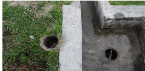
Figure 6. An air vent made of concrete is broken
