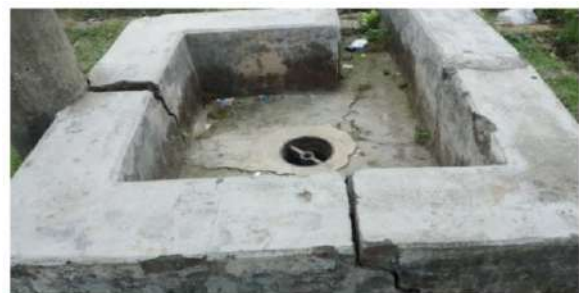
Figure 7. Cracks in the CC structure around the outlet
