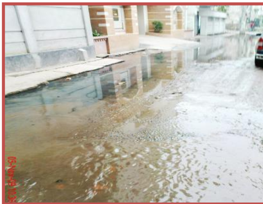
Source: Field Survey, July 2010 Fig. 5: Permanent water logging in road
