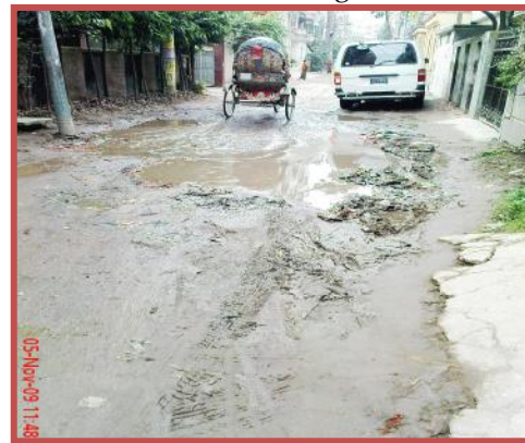
Source: Field Survey, November 2009 Fig. 6: Broken roads
