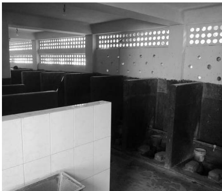
Fig. 3. Toilet in Bandar Mosque.
