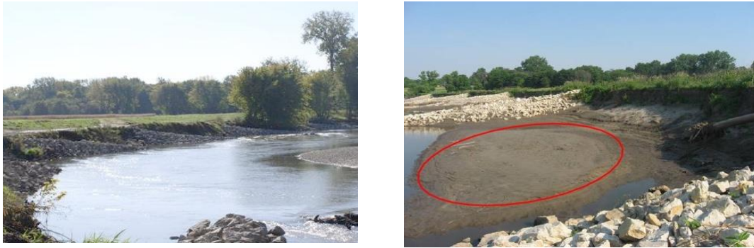
Fig. 1. Photographic view shows the series of stream barbs installed along the river bank during flow season (left-hand side) and low flow season (right-hand side). The red circle indicates sand bars formed after installation of barbs.
