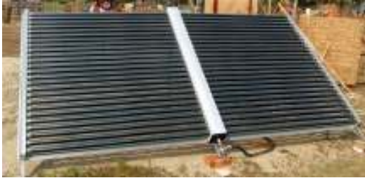
Figure 2. Evacuated tube solar collector used with the paper drier.
