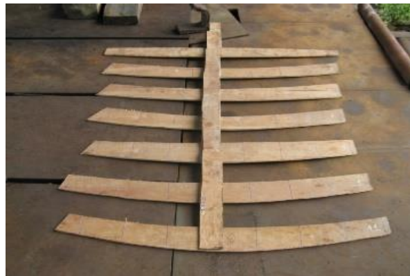
(c) Fabricate the templates at the test positions according to their dimensions on the drawing
