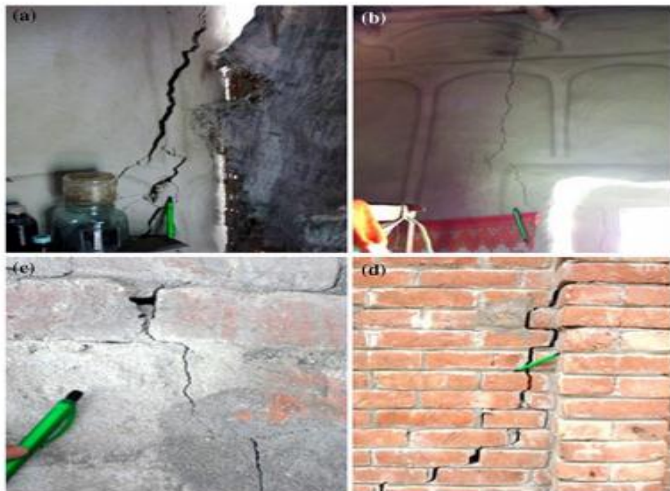
Fig. 7. Subsidence impact on structures. For example, these representative photographs showing the effects of land subsidence on mud wall (a and b) and brick wall (c and d) around the Barapukuria coal mining area [6].
