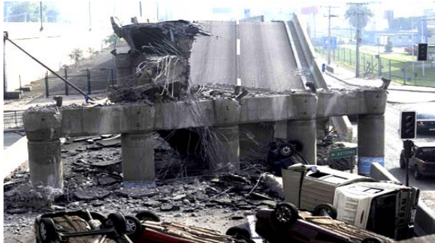
Fig. 8. Earthquake related catastrophic failures in structures reinforced with brittle steel bars.
