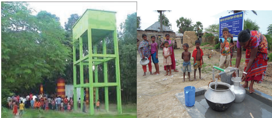
Figure 4: Deep tube-well water supply installation (DTWSI) system
